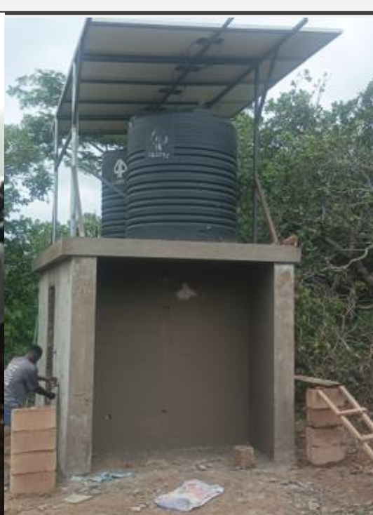
Figure 2: Solar-Powered Water Reservoir System at ACET UNDP GEF-SGP CSALC, Agbada 2
